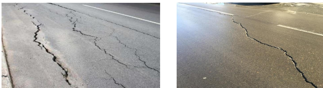
Fig. 2. Disruptions (depth) and cracks caused by deformations in the base layers of the road surface.
